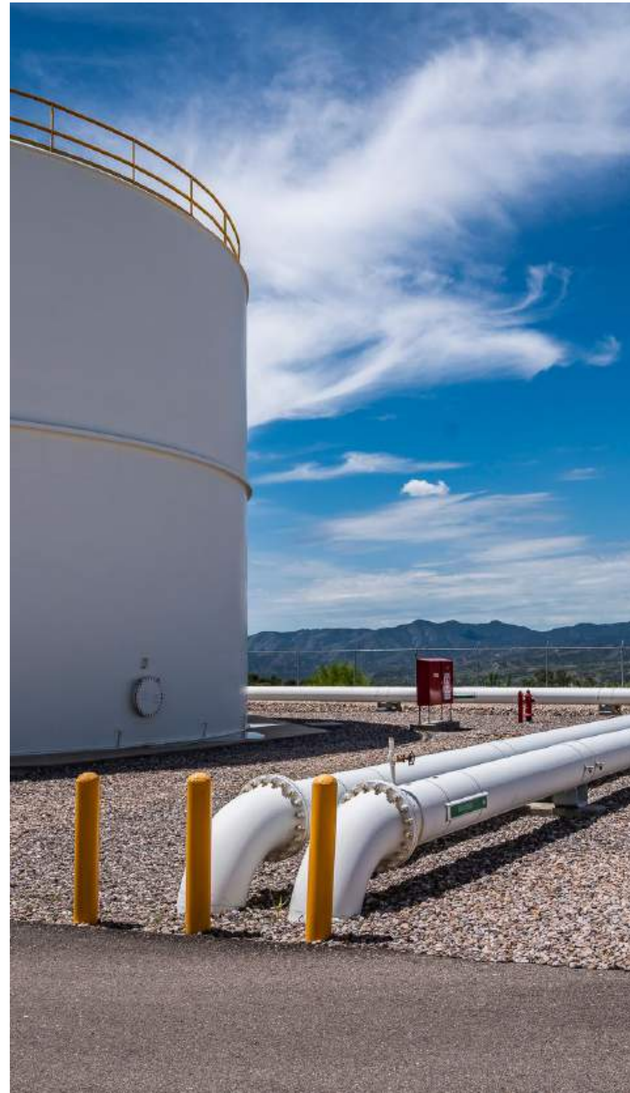
Combined Cycle Plant, Sonora, Mexico
