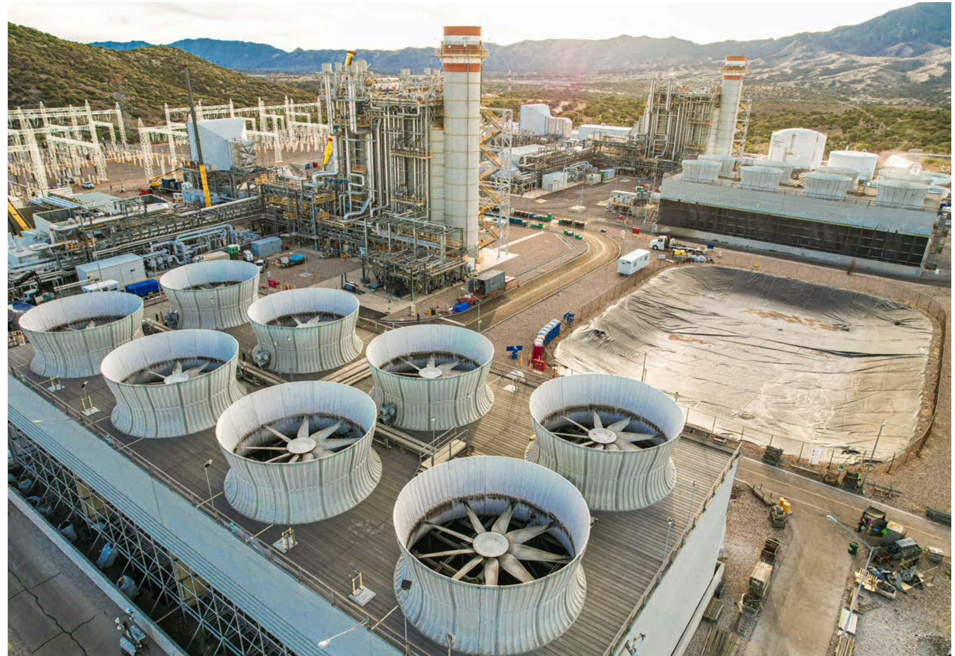
Combined cycle power plant, Nacozari de Garcia, Sonora México
