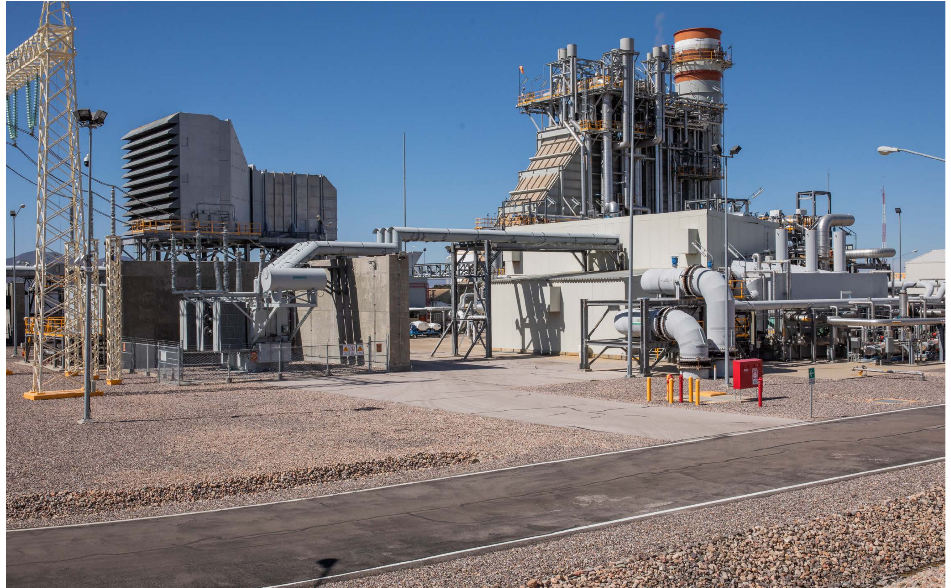
Combined cycle power plant, Nacozeni de Garcia, Sonora, Mexico
